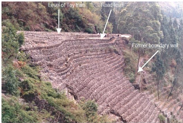
Figure 8 Subsiding Hill-Cart road al Lower Pagla Jhora. The Toy train and the vehicular tracks are at different levels. The former boundary wall of the road is found at a lower level (Photo: S. R. Basu)
