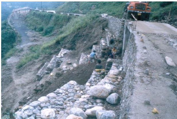
Figure 9 Building the retention wall along the Hill Cart road at Pagla Jhora without any weep hole (Photo: Author)
