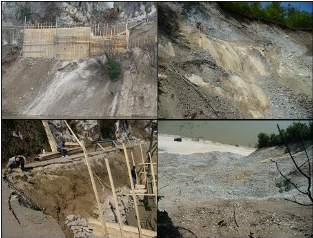
Fig. 4: The collapse of Mraconia and the landslide of Liubotina
