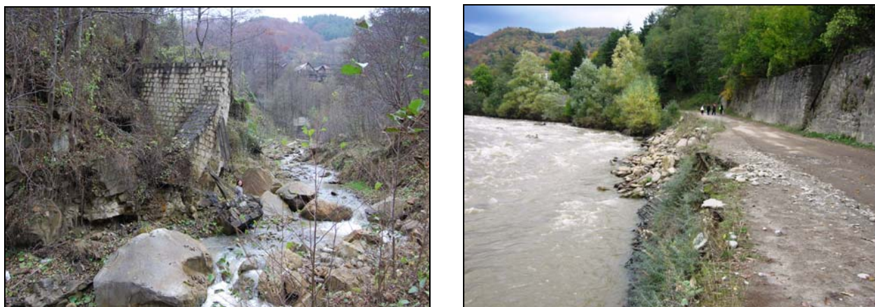
Fig. 7. Economic damages caused by the fluvial dynamics processes: a – degradation of hydrotechnical works in the Păltiniș River channel; b - erosion and crumble of the departmental road DC178 near auto-station Varlaam) (Photo: Minea, November and July 2009).
