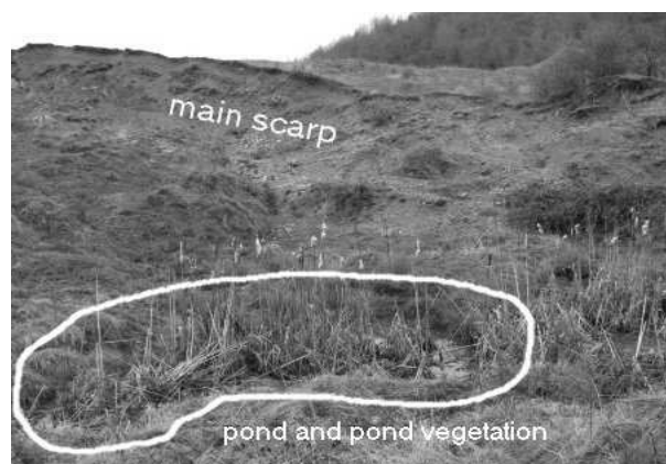
Fig. 6. Poned water on the head of a landslide
