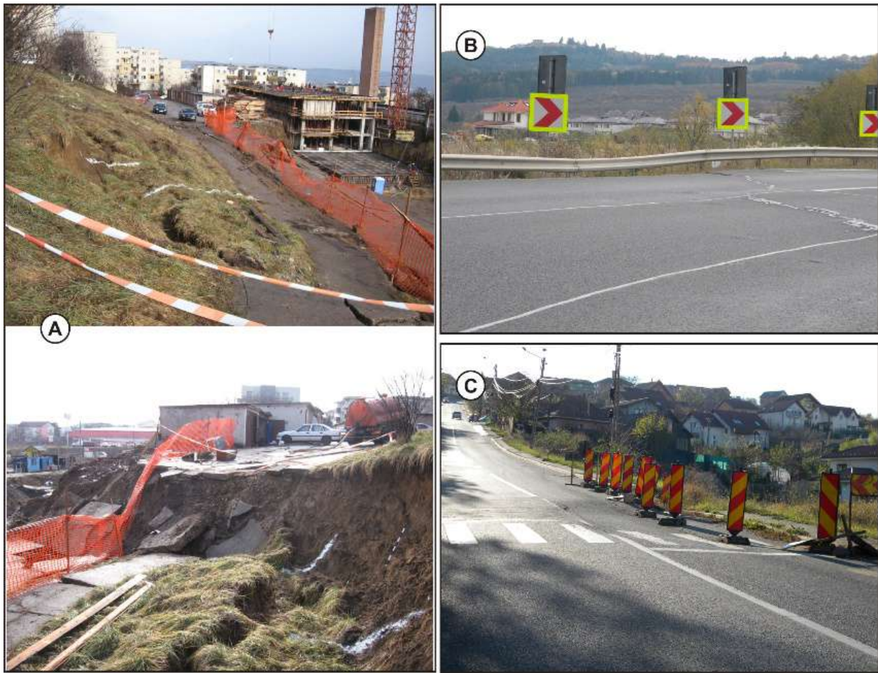
Figure 10 Landslides caused by constructions (A) and affected the roads (B, C)
