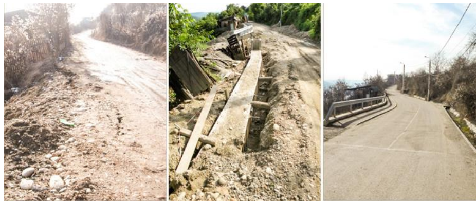
Figure 10 The restoration of Uliului Str., Grigorescu neighbourhood (Left and middle: large fractures on the street; Right: the consolidated road which is still under risk of sliding)
