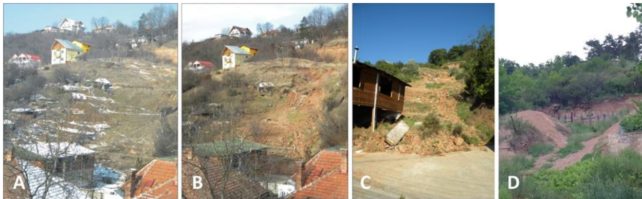
Figure 8 The reactivation of mass movements on Dragalina Str., Grigorescu neighbourhood (A: the area under dry conditions; B: mass movement reactivation due to constructions and high water content in soil; C and D: the continuous mass movement) (source of Fig. 8A and 8C: Poszet, 2017)
