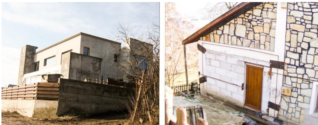
Figure 11 Attempts to repair cracked buildings (Left: alternative concrete structures used to stabilize the building; Right: improvised methods used to hold a house together)
